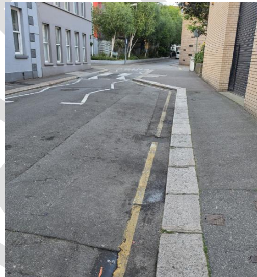
View towards Hilgrove Street junction – shows area where asphalt is breaking up.
