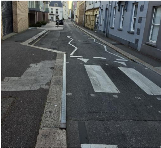
View towards Peter street – uneven surface and breaking up in areas.
