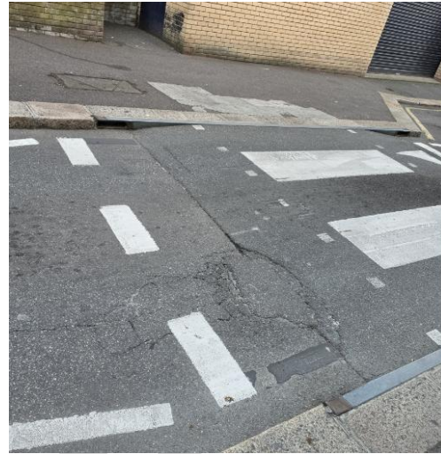
Road surface breaking up in front of the speed hump.
