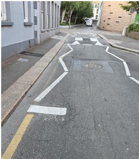
View towards Hilgrove Street junction – shows area where asphalt is breaking up.
