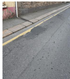
Temporarily plugged pot holes, further deterioration of the road surface is occurring.
