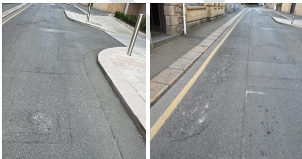
Various potholes are beginning to form.
