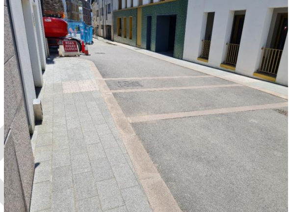
View from Nelson St Car Park, standing on the east footway looking southwards to Minden Place
