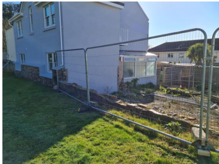
Photograph : The property 'Bow Cottage', showing the demolished party wall that formed part of the property's rear wall.
